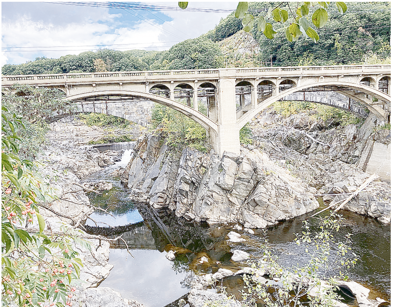
The Vilas Bridge in Bellows Falls at the Great Falls and directly over the petroglyphs, which was the geographic center of the two-year Kchi Põntegok Project to document, catalog, and study Native culture.
