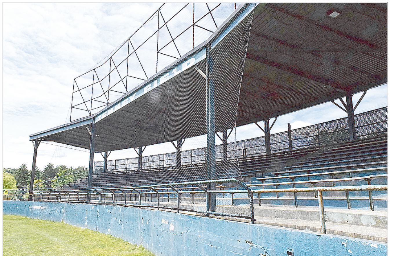
The grandstand at Tenney Field in Brattleboro, closed to fans since 2017, is set to get some much needed repairs and upgrades this summer.
