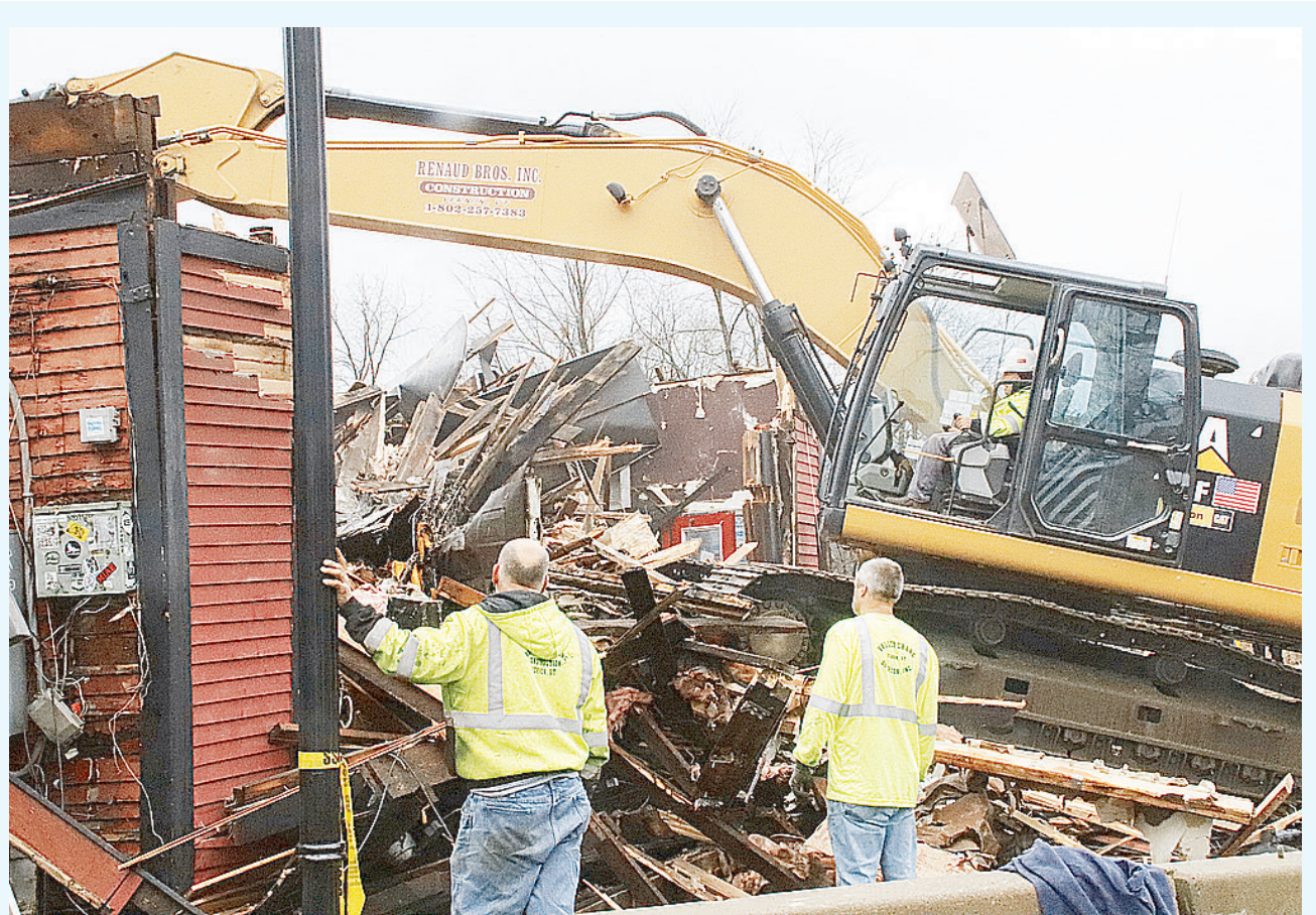
Workers from Renaud Bros. in Vernon demolish the remains of the McNeill’s Brewery on Dec. 3, 2022.
